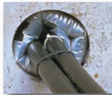
Power Cable Feedthroughs
