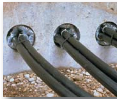
Power Cable Feedthroughs
