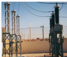
HV Surge Arresters
